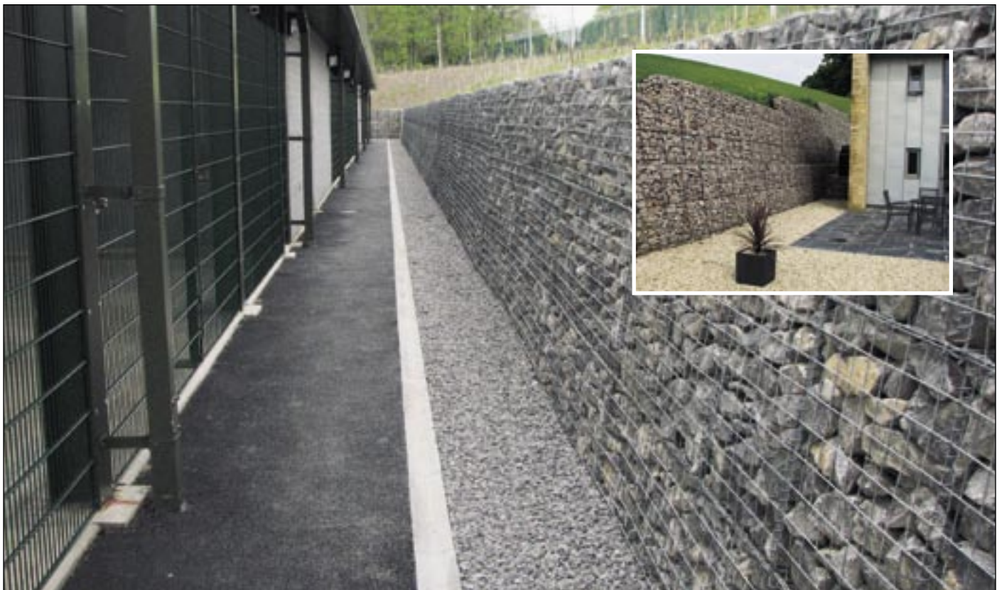
▲ Mass gravity gabion wall designed and constructed with a flush face at Catterick Garrison.
