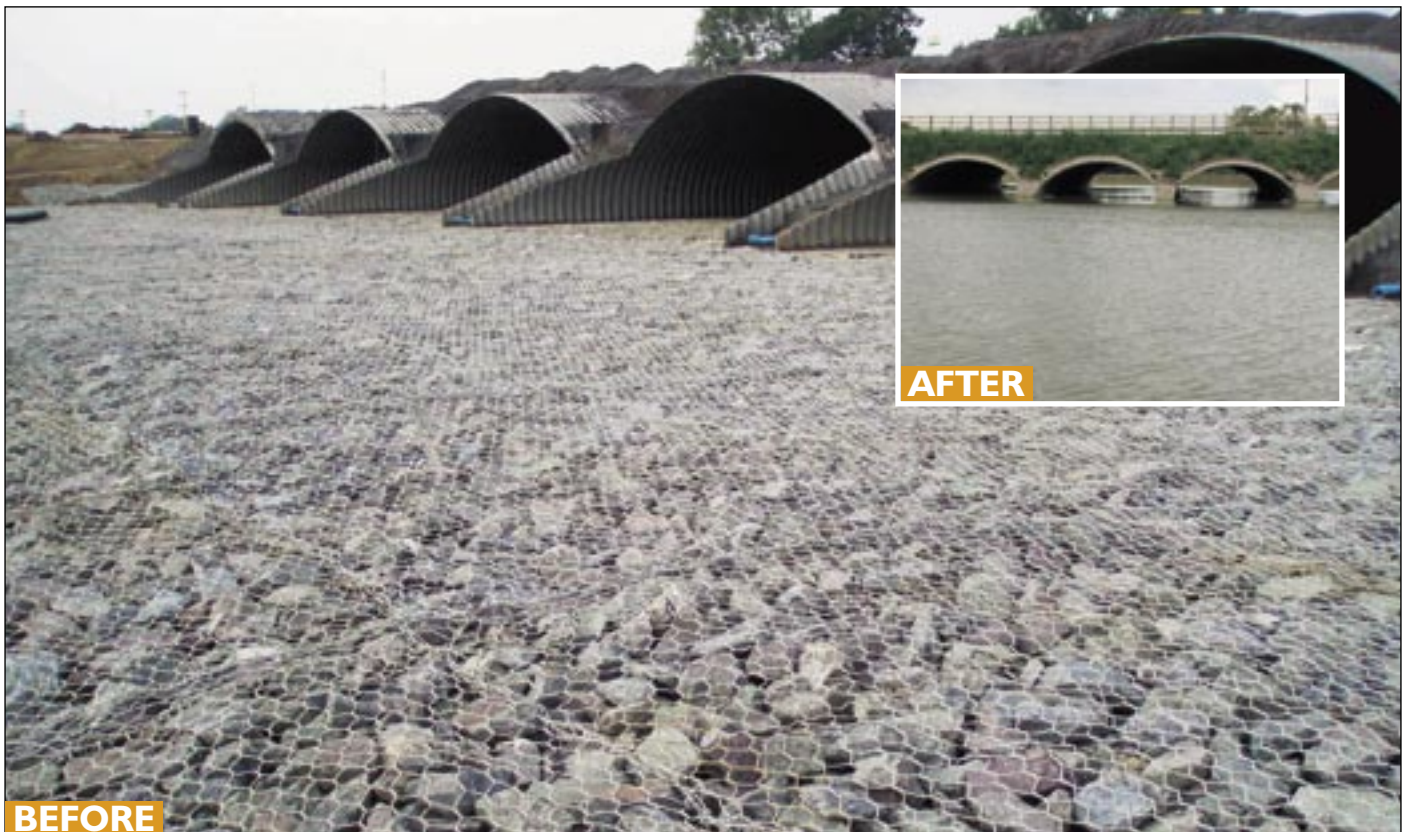
▲ Hexagonal woven wire mattresses acting as an erosion protection apron to a new lagoon at Swann Valley, Northampton.
